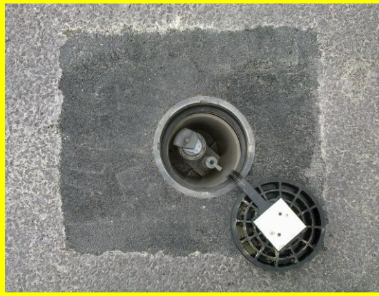
Premier Boundary Water Meter Box in service.
